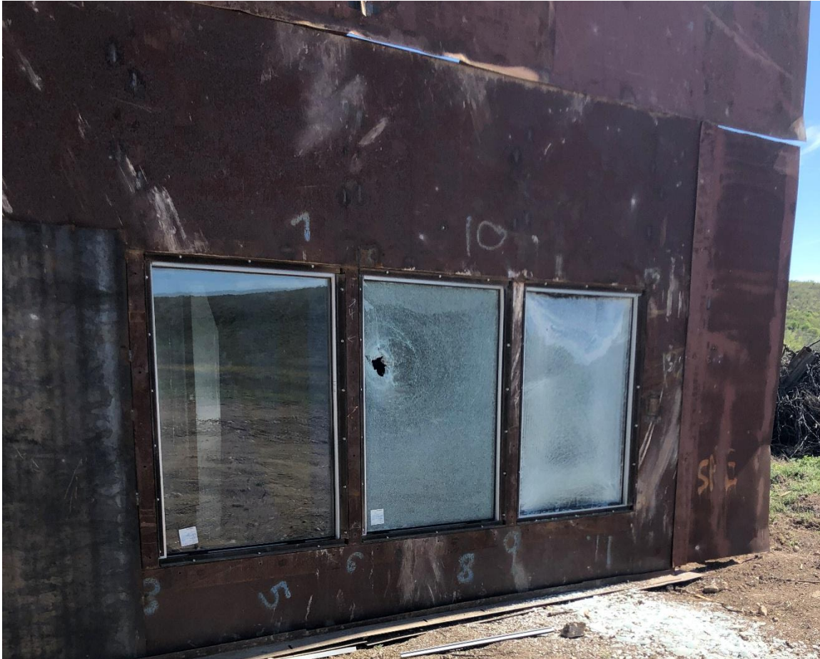
Photo No. 8 Post-test Specimen 27, 25, 26 exterior
